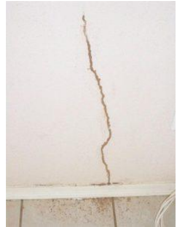
Termite mud tubes
