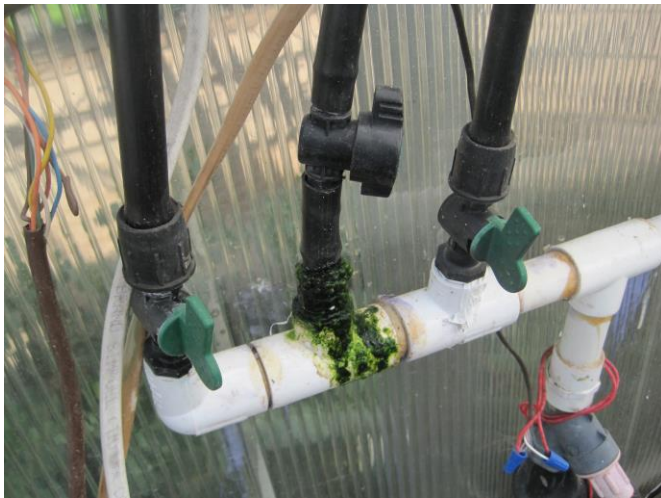
Figure 1: Algae clogging irrigation lines. Photo by L. Pundt
